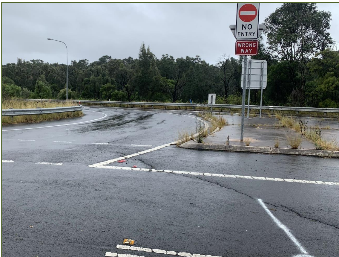
Figure 2.0.1 – Diagonal Cracking near Princes Highway Off-Ramp
