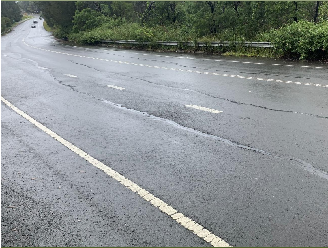
Figure 2.0.4 – Sealed Longitudinal Cracking
