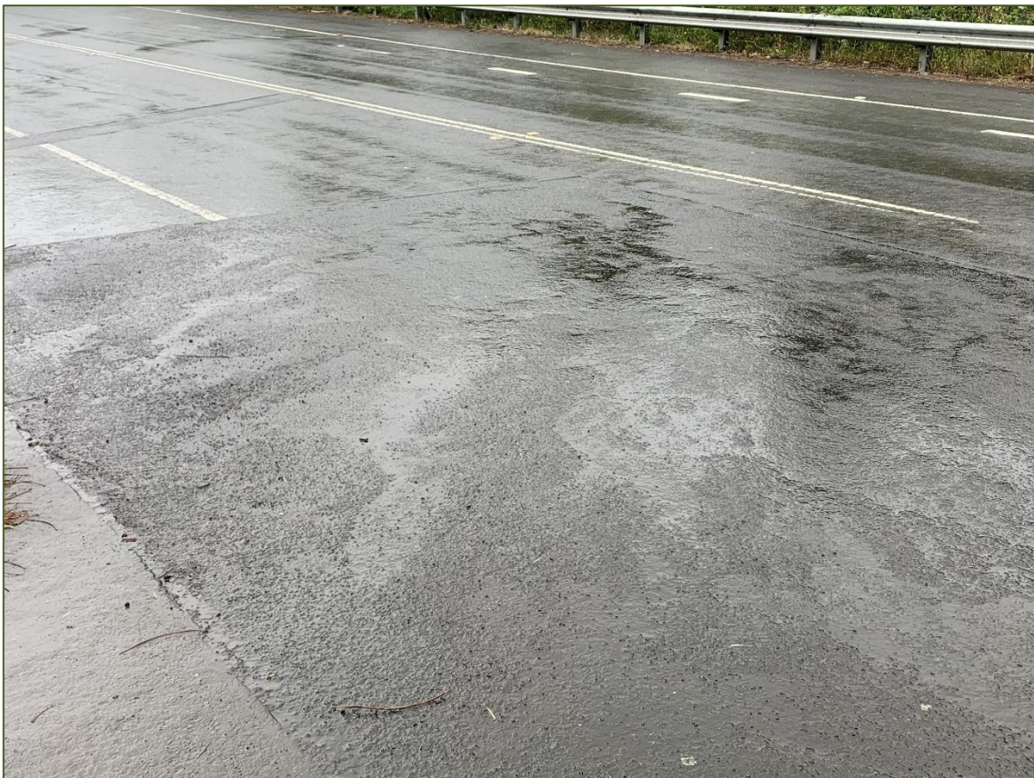
Figure 2.0.5 – Patching and Minor Deformation
