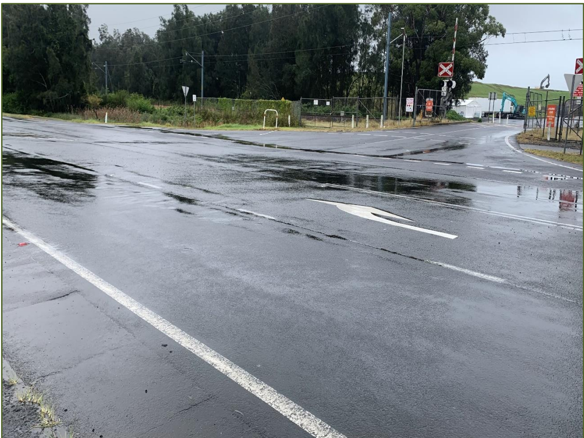
Figure 2.0.9 – Minor Rutting (Entrance of Kiama Community Recycling Centre)
