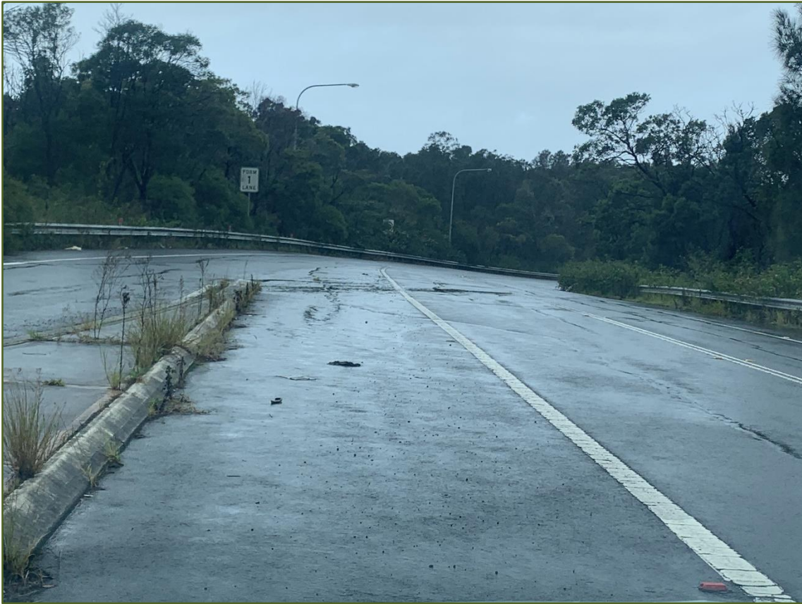
Figure 2.0.2 – Minor Longitudinal Cracking
