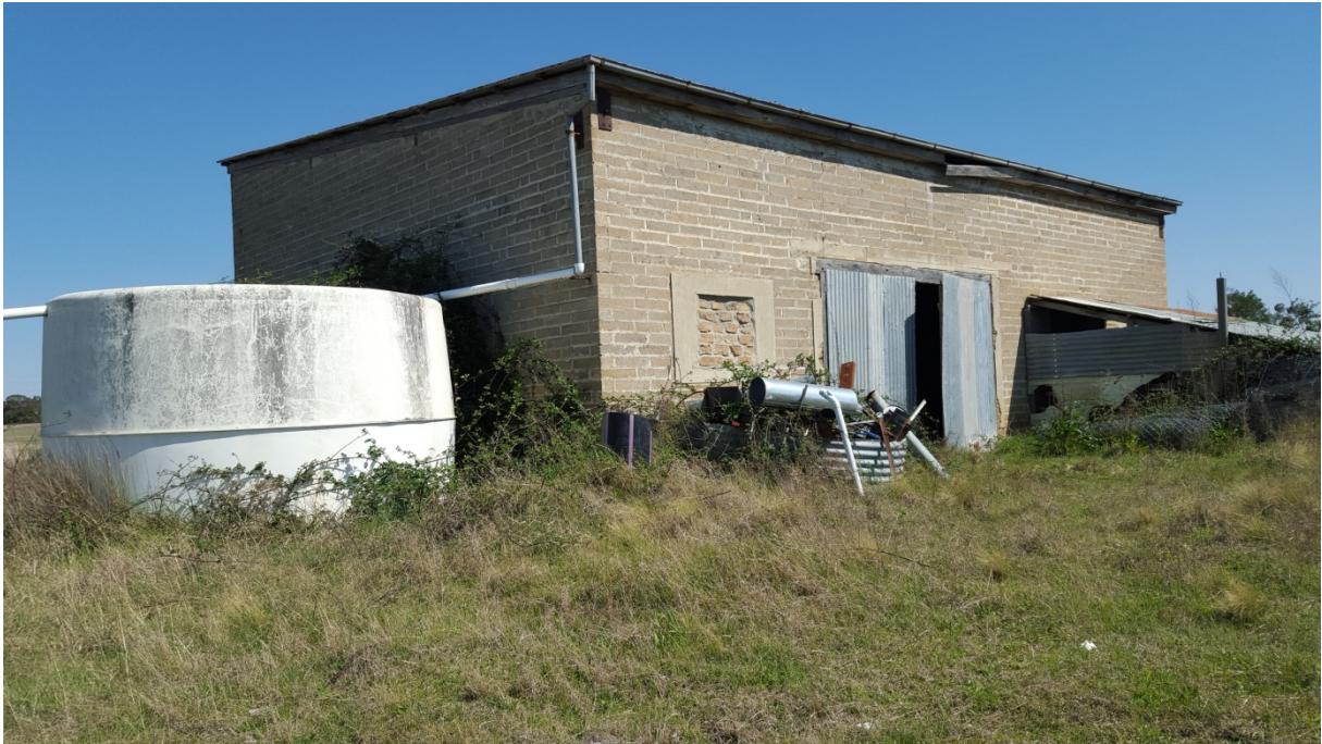
Plate 3.12 Rear of the control room showing corrugated iron engine housing, doors, bricked in openings and a water tank (20151006_145129).
