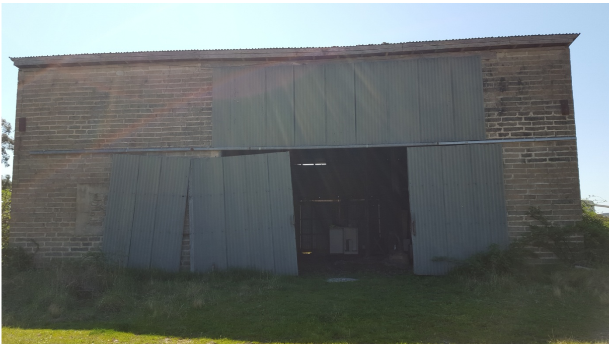
Plate 3.11 Front of the control room (MS04_11), facing west, showing the corrugated iron rolling doors which would have opened to let out heat (at the base) and for the rope to rotate (top) (20151006_144642).
