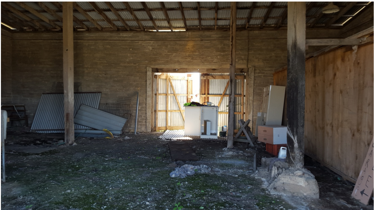
Plate 3.13 Interior of control room showing wooden beams for piles and roof, concrete foundations and dirt floor (20151006_144957).
