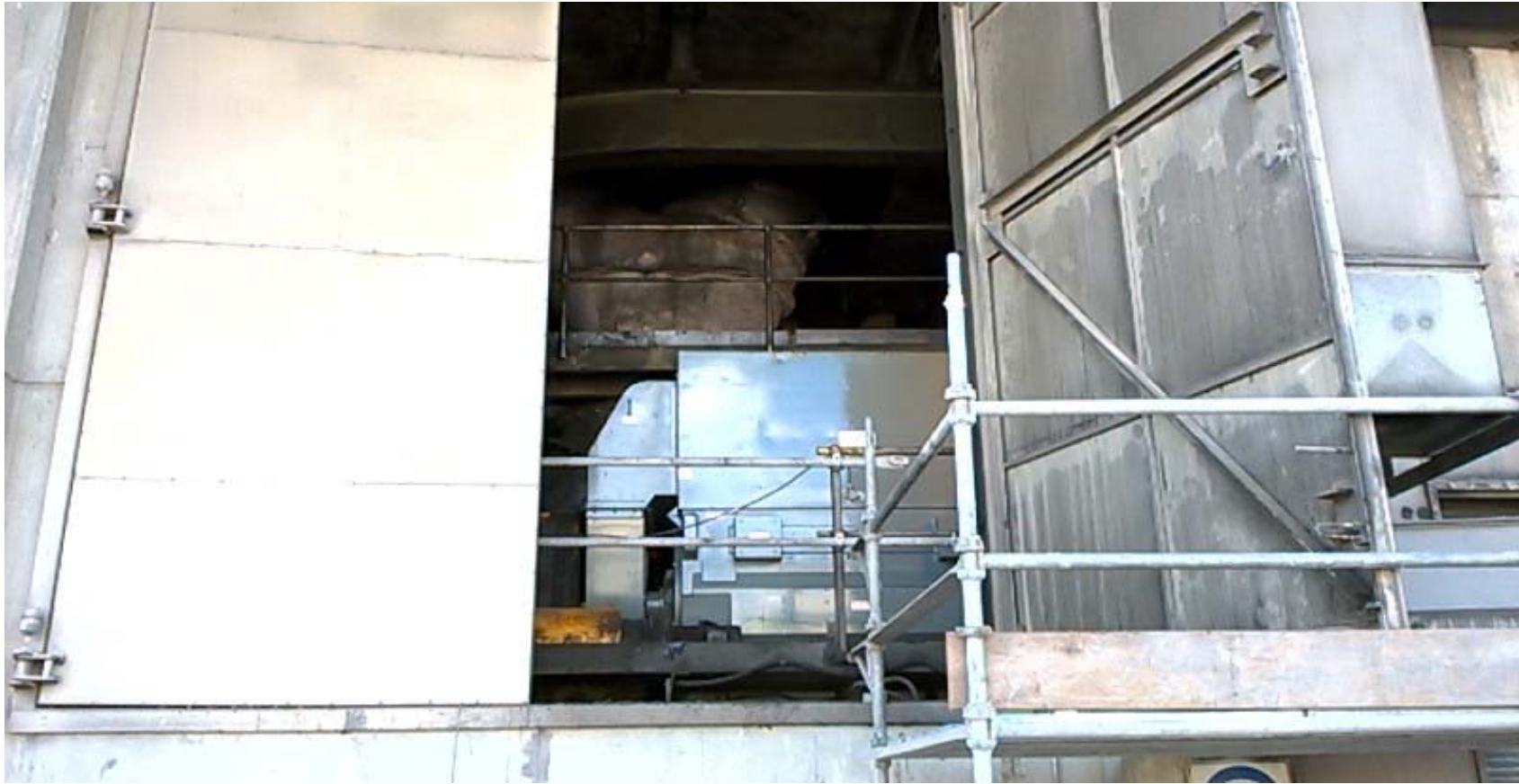
Figure 3.5: Coal Mill fan room door open, southern side of Coal Mill Building
