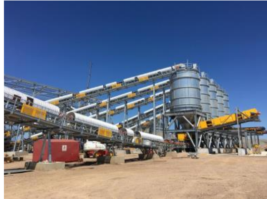
New product silos and blending plant at Deer Park Quarry, Victoria
