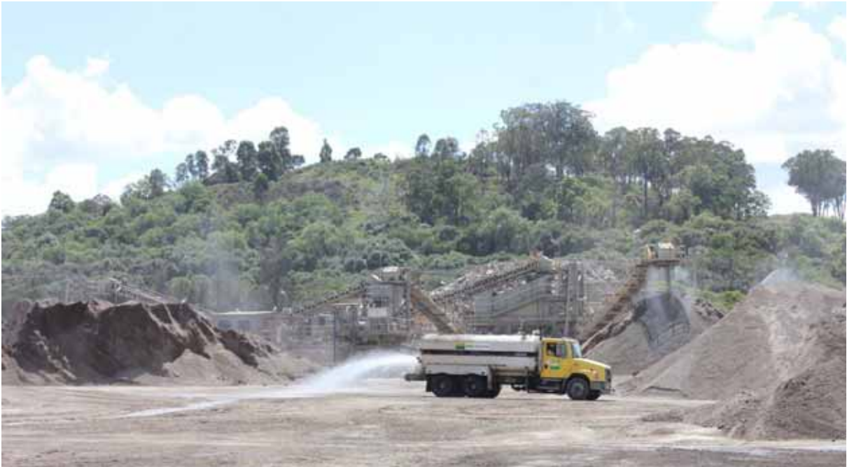
Photograph 14.3 Photograph taken within the site showing processing plant in the foreground and existing vegetated ridgeline immediately north of the facility which provides visual screening
