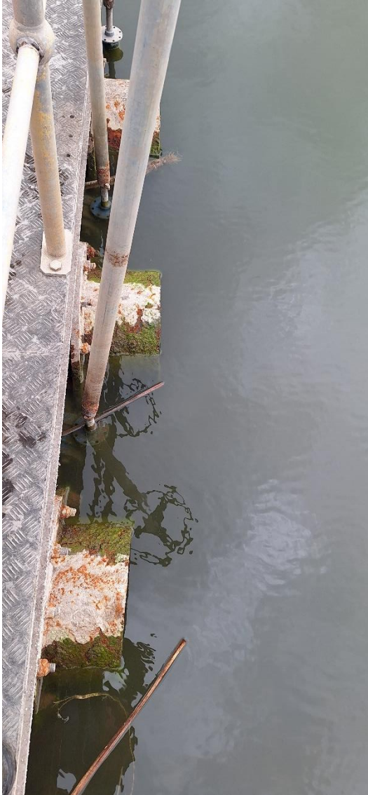
Plate 2 – Discharge Pipes in with Valves in Closed Position
