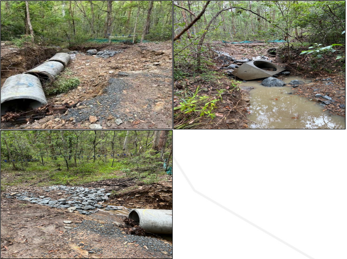
Photo set 5: Damage to crossing, dated 8 January 2024.
