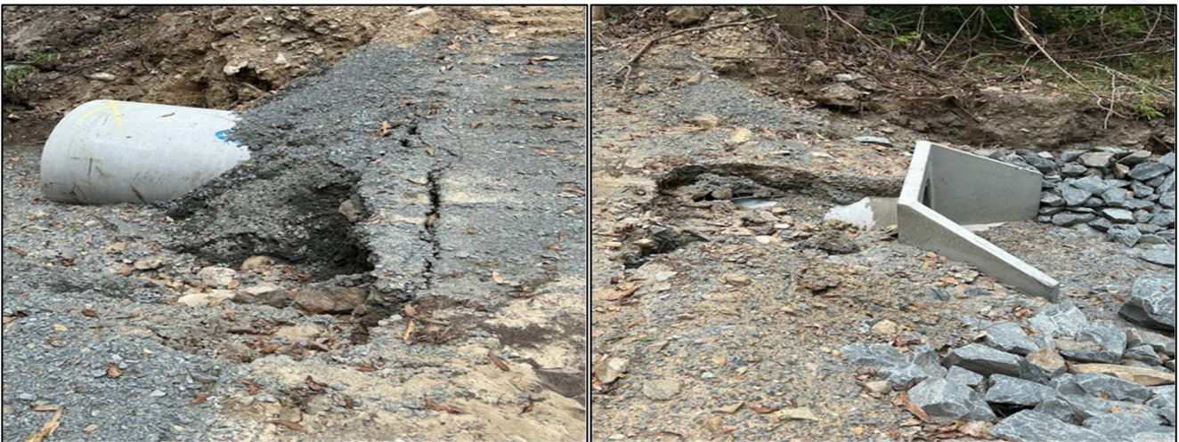
Photo set 4: Washout at headwall, photos dated 19 December 2023.
