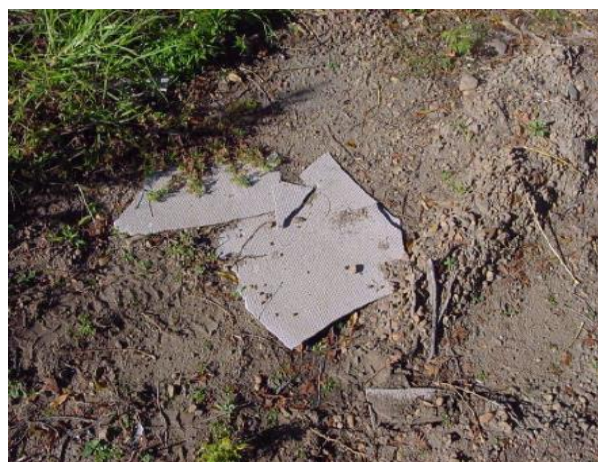
Photo 6 – Fragments of Asbestos Cement sheeting on ground surface
