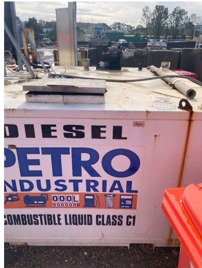
Photo 16: Diesel Storage (19 August 2025)
