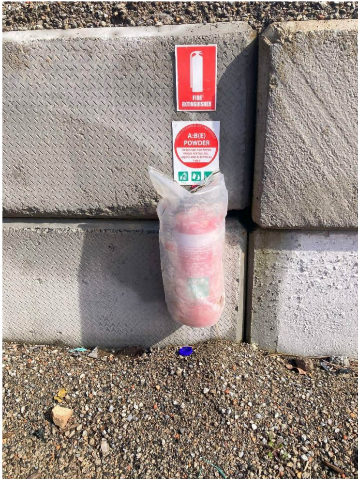
Photo 17: Fire Extinguisher (19 August 2025)
