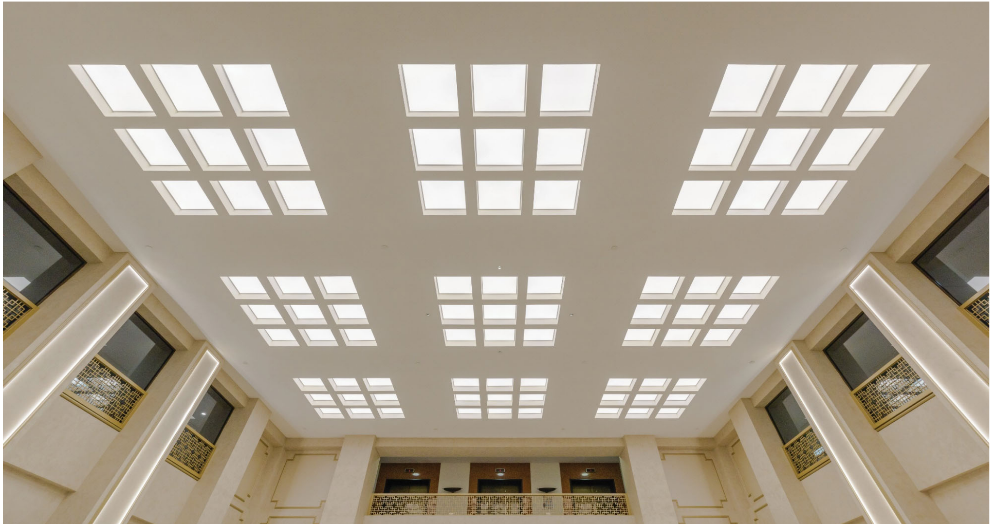
USG Boral Ensemble® Monolithic Acoustical Ceiling, Chancery House, Western Australia
